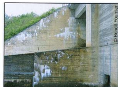
Figure 2 – Alkali-reaction on the hydro-electric dam of Hunderfossen (1964)
