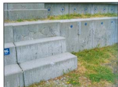
Figure 1 – Concrete distress in the Lillehammer Olympic Park (1994)
